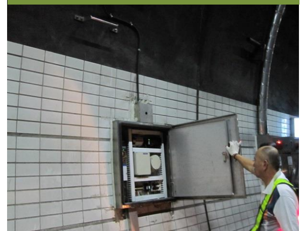
Local panel / sensors
