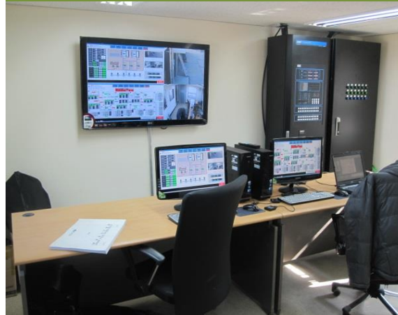
Local Control room
