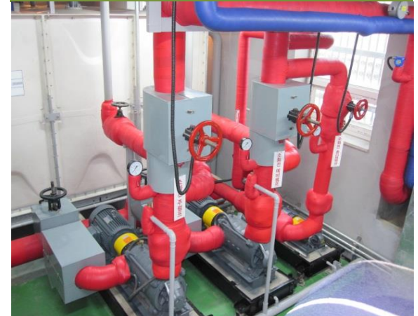
Hydrant pump & Tank
