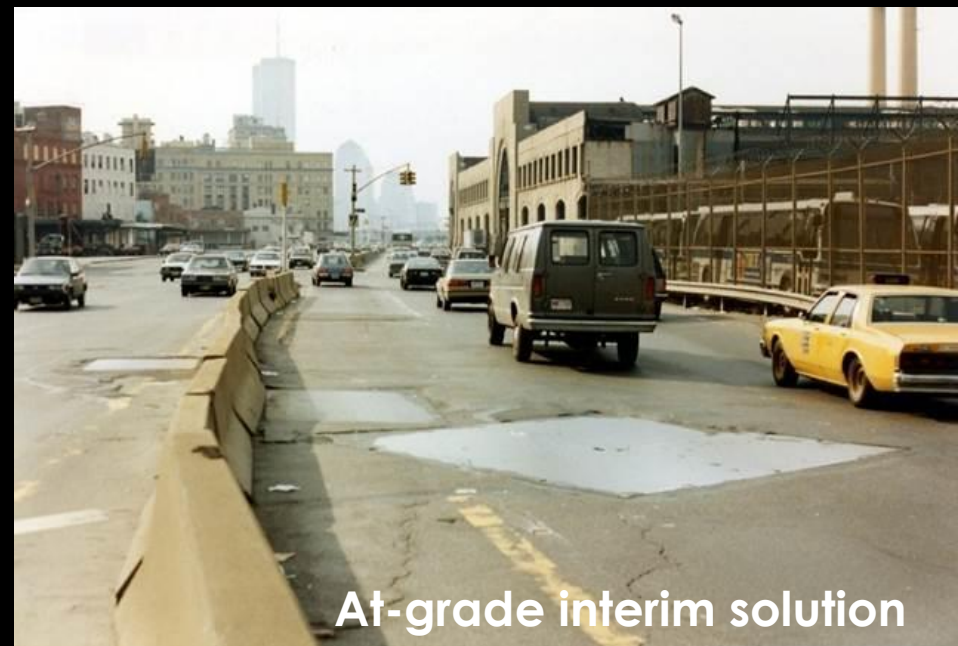
Post Highway Collapse
